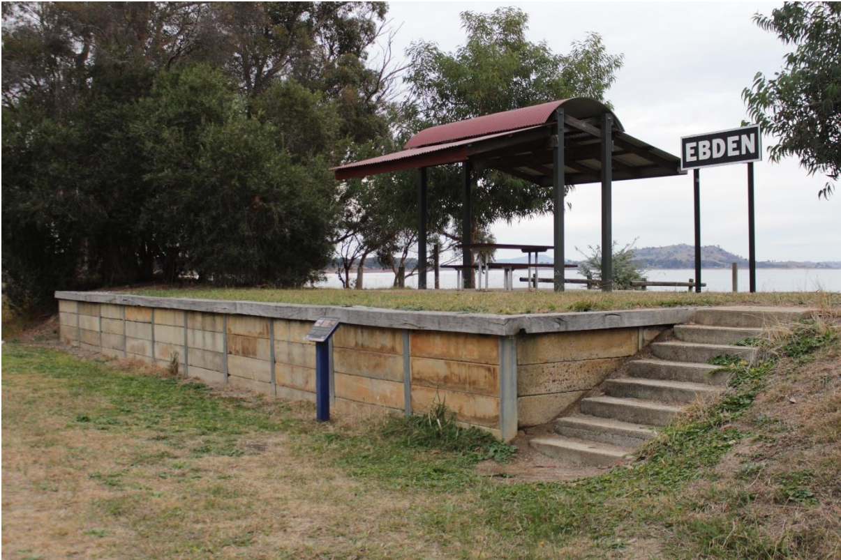
Ebdon Station showing retaining walls, timber edging and concrete stair (RBA, June 2024)
